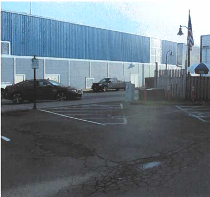
Fatigue Cracking – Abbey Street Lot (2016)
