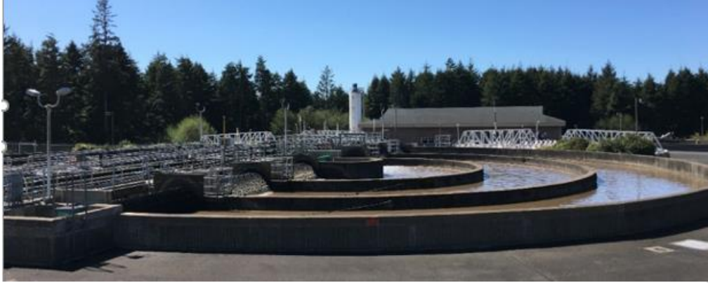
Aeration and Settling Tanks at the Vance Avery Wastewater Treatment Plant
