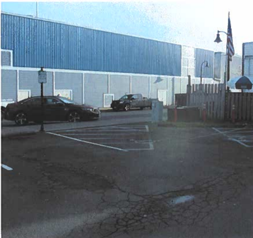
Fatigue Cracking – Abbey Street Lot (2016)
