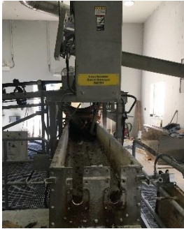
Thermoblender at the WWTP- Used for Pasteurizing Class A Biosolids
