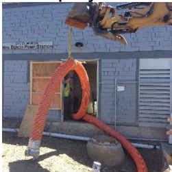
Nye Beach Pump Station
