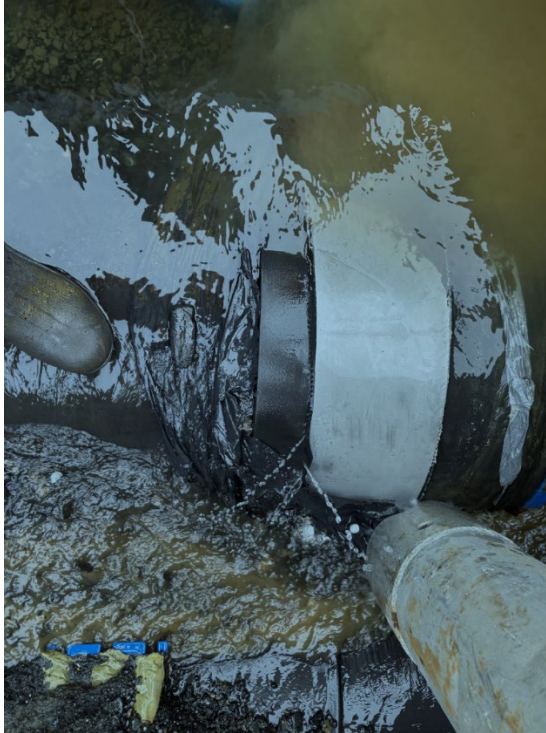
Discovered leak, Dec., 2024
