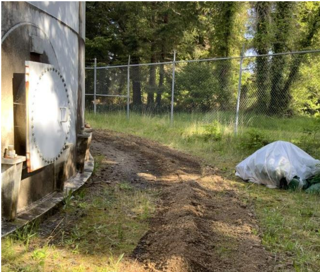
Cathodic Protection at Yaquina Heights Tank
