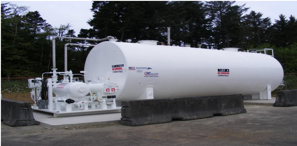
Jet A 12000 Gallon Fuel Tank- Airport
