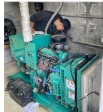
WWC crew checking lift station generators
