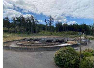
WWTP Aeration Basin
