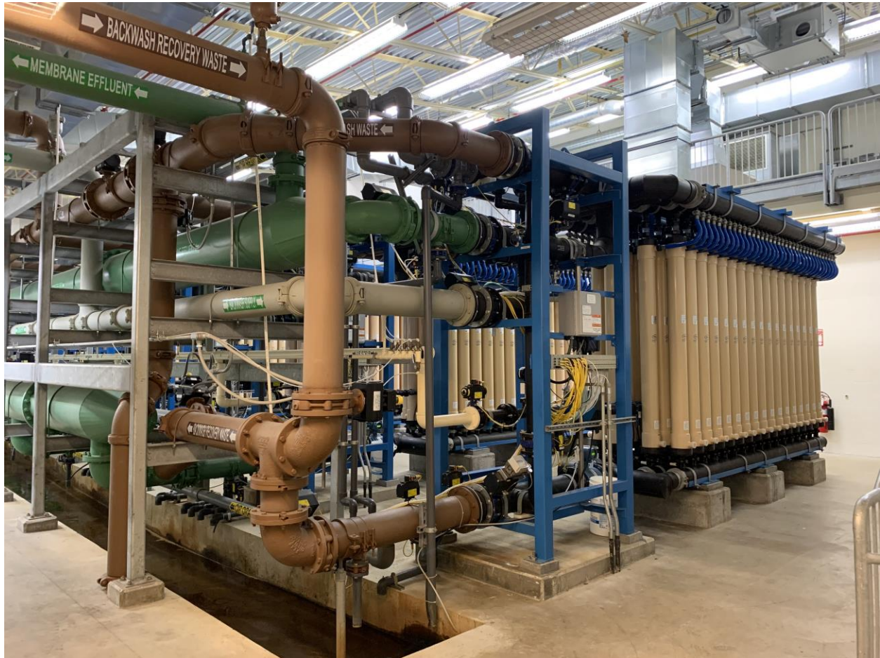
Water Treatment Plant Filtration System
