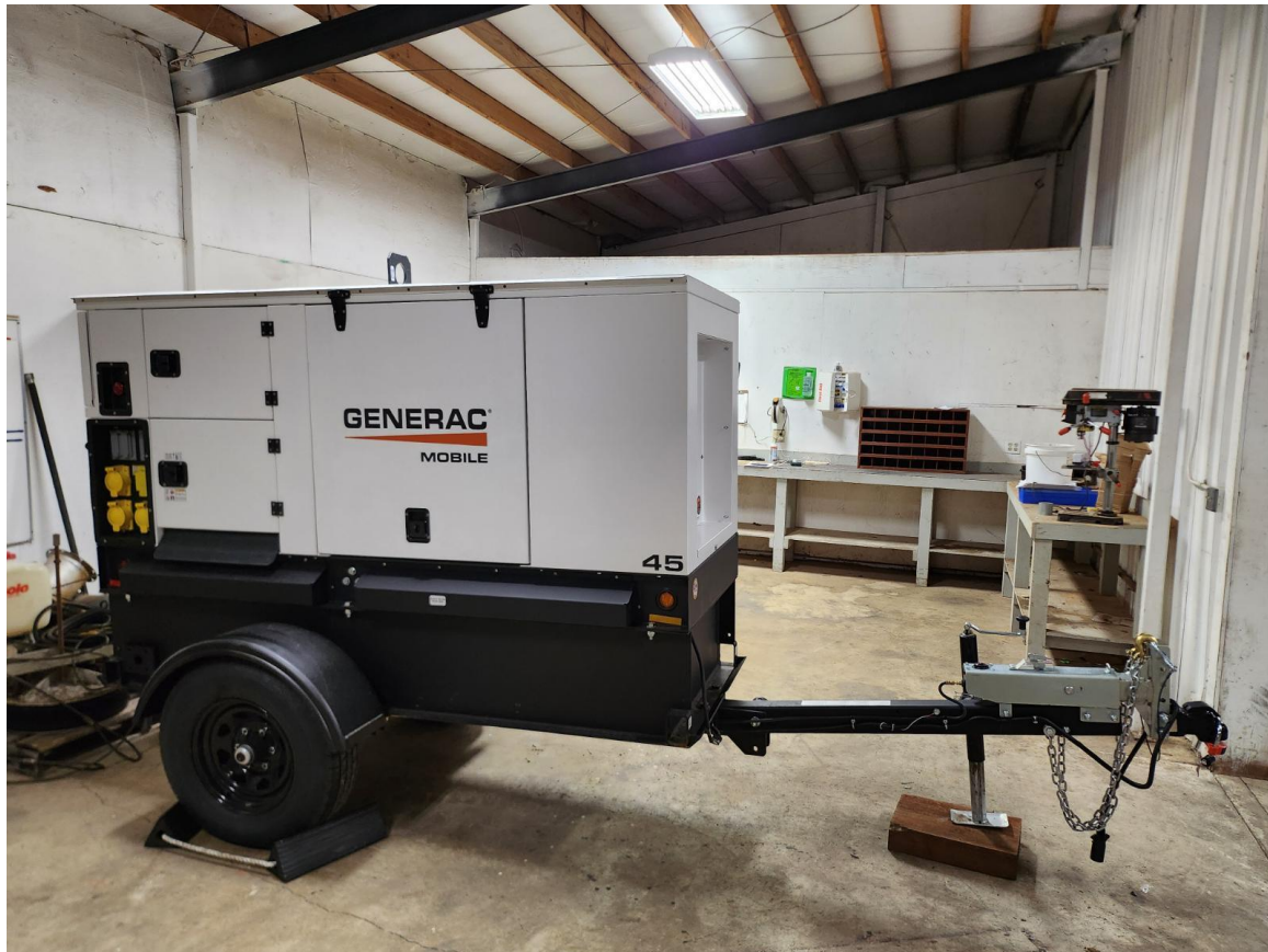
Mobile Generator for the Wastewater Treatment Plant
