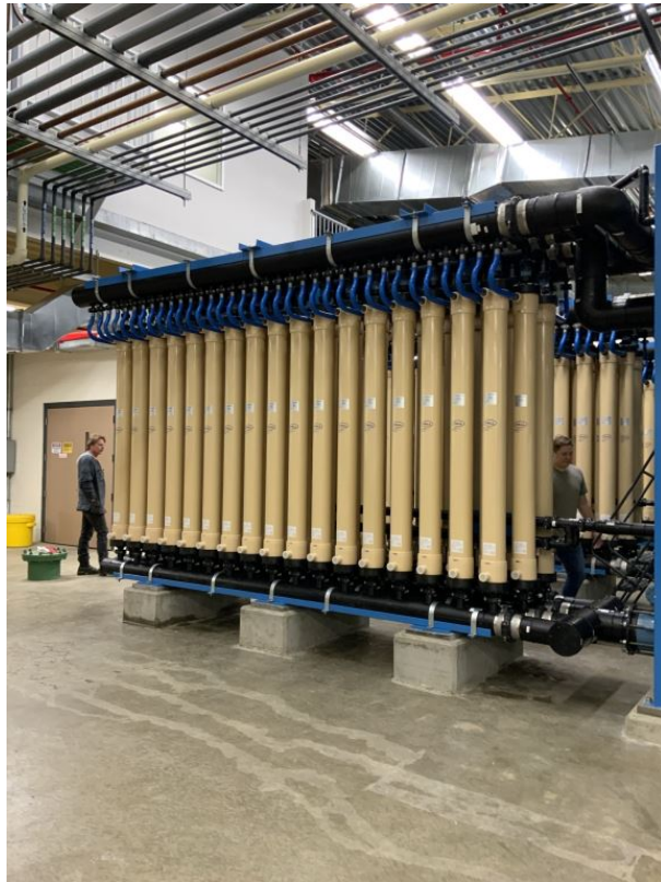
Water Treatment Plant Filtration System
