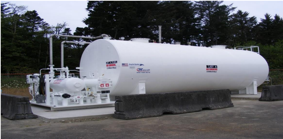
Jet A 12000 Gallon Fuel Tank- Airport
