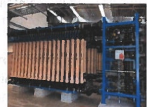
New Water Treatment Plant Filtration Rack
