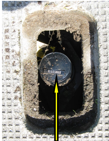
Take off the metal lid to reveal the water meter. You might need to remove some dirt to get to it. That number is your water meter number.
