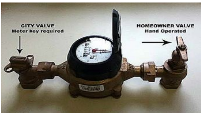
On the left is a typical water meter setup with a homeowner shut-off valve installed. Again, you will probably have to remove some dirt to find it. This photo is an example, and your valve may look different, but it will be between the water meter and the residence. This valve is useful if you need to turn off the water to your house. City ordinance now requires the installation of this valve; if you have an older house, you may not have had one installed. We encourage you to get one installed by a plumber. Don't wait until it's the middle of the night and you are dealing with a broken water pipe!
