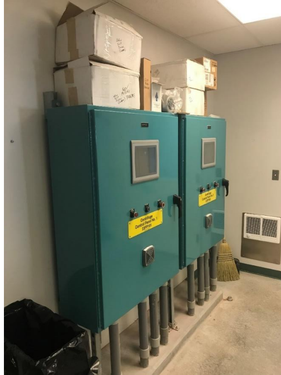
Figure 8: Existing Centrifuge Control Panels
