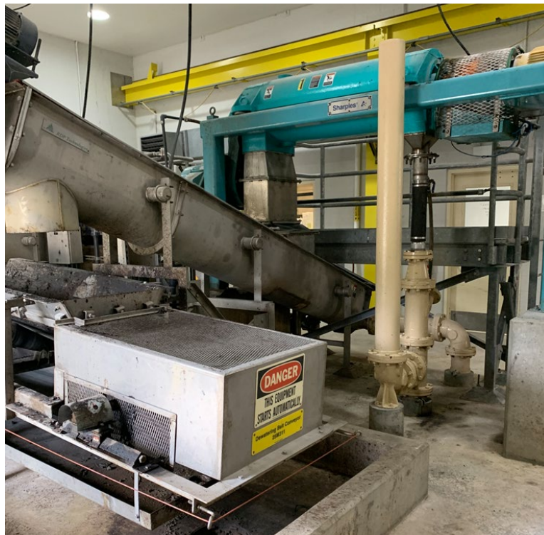
Figure 7-7. Existing dewatering centrifuges
