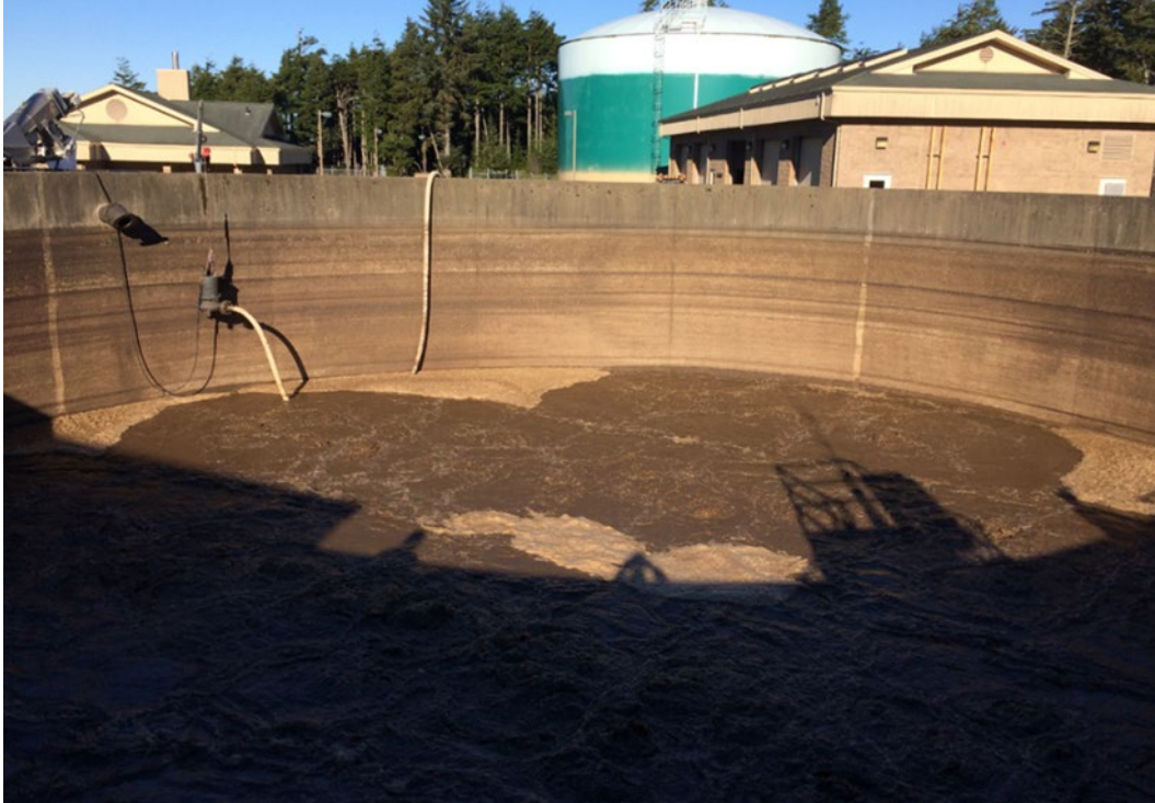
Figure 3-3. WAS storage tank
