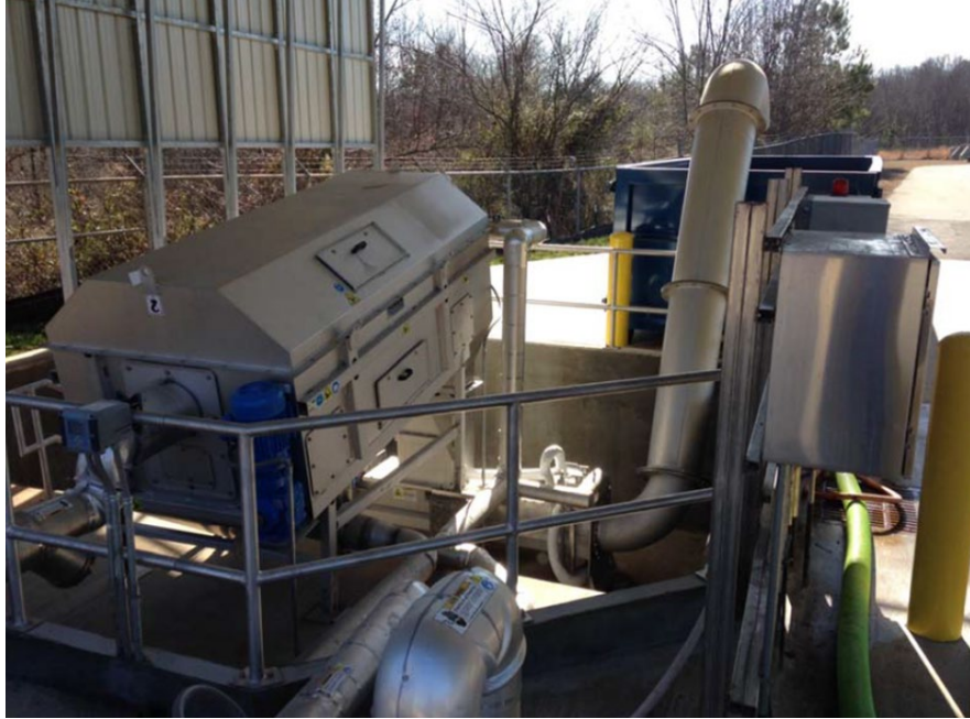
Figure 7-1. Huber RoFas packaged hauled waste system
