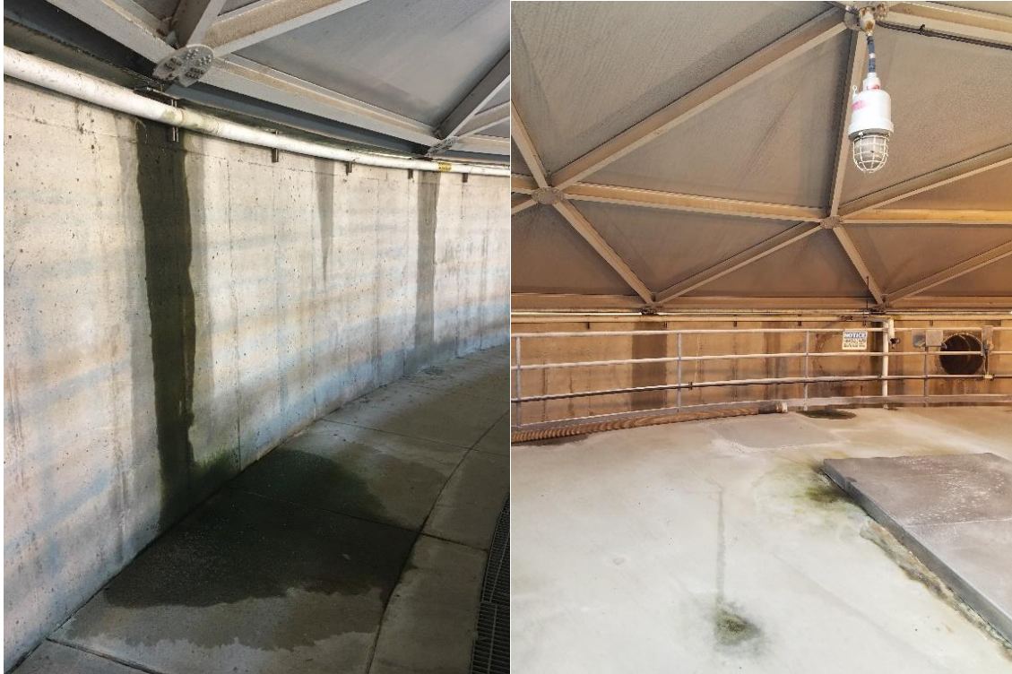
Figure 2. Examples of rainwater leakage through geodesic dome
