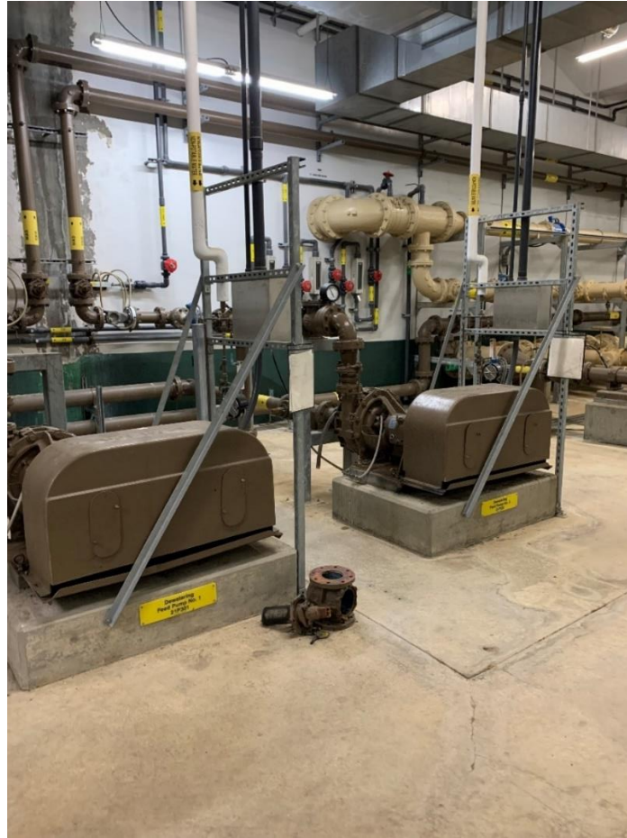
Figure 9: Dewatering Feed Pumps
