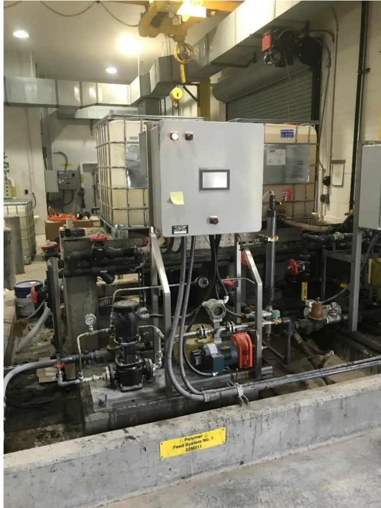
Figure 11: Existing Dewatering Polymer System
