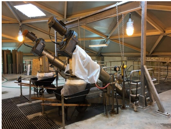
Figure 4. Existing Auger Screens
